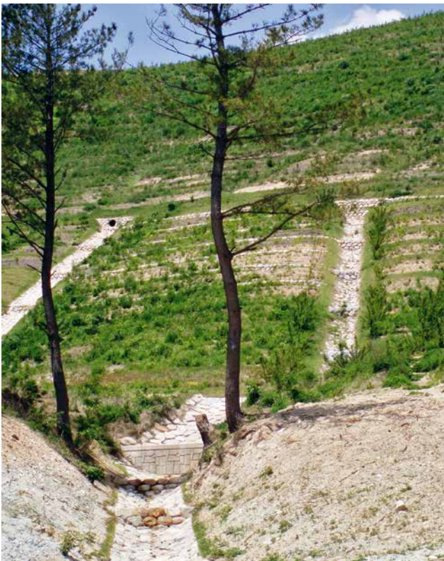
Hillslope restoration in Korea. Harsh conditions (eroded soils, droughty sites) required restoration using a combination of physical water control structures to control erosion and tree planting. Photo © John Stanturf
