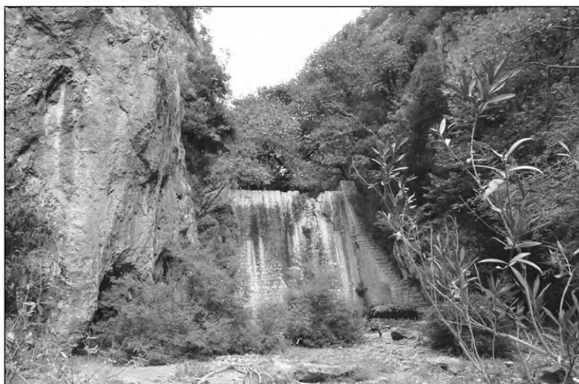
Figure 4. View of a damn in Nedon river; a major part of its basin was burned during the summer of 2007.
