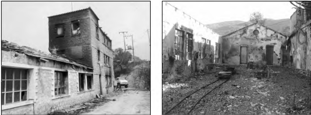
Figures 2a and b. External and inside view of the timber sawmill after the fire.
